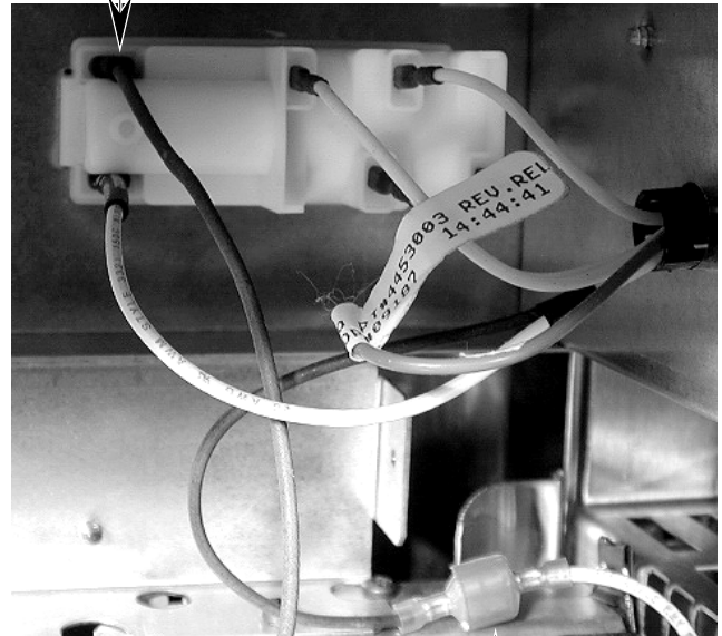
Ignition Switch Wire Connector At Spark Module
