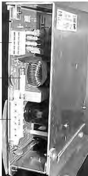
10 PIN PLUG (C 10) SPEED CONTROL BOARD FUSE (See NOTE Page 52) 6 PIN PLUG (C 6) SPEED CONTROL BOARD
