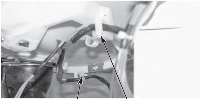
Motor Control Unit Wiring Standoffs
