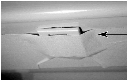
Door Switch Taped Closed
