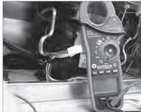
Measuring compressor motor resistance
